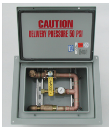
Emergency Oxygen Inlet Box
