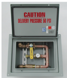
Emergency Oxygen Inlet Box
