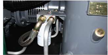
Lubricant filter assembly features a spin-on, full-flow, 12µ, high-efficiency element.
